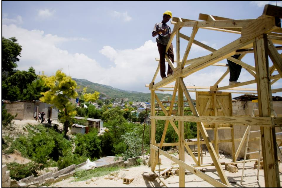
CARE staff and community volunteers work together to build transitional shelters in Carrefour, one of the hardest-hit communities in the Port-au-Prince metropolitan area.
