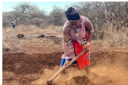
Nonkota Kaleiya constructing the earth miles in Alooca conservancy ,this technique is important in restoring rangelands Photo credits Faith Tanui WWF-Kenya -Kenya
